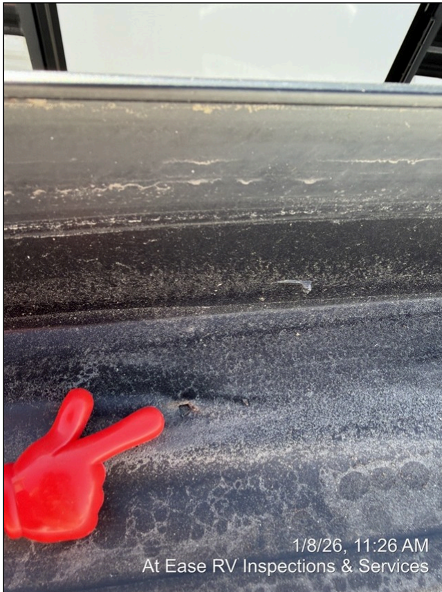
9.2 Item 3 (Picture) Gap in tape
