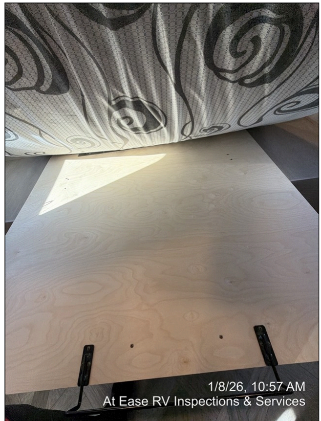
21.6 Item 2 (Picture) Under bed
