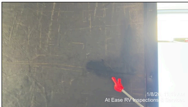
9.4 Item 3 (Picture) Stain on the slideout floor
