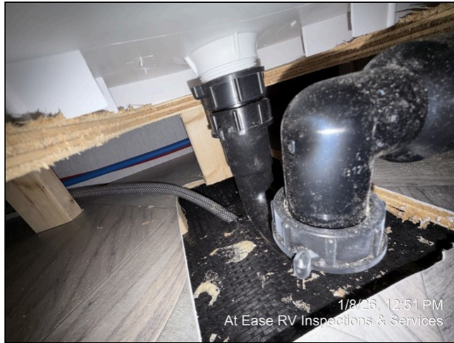
19.17 Item 2 (Picture) Under shower
