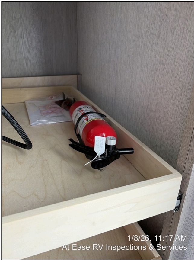
5.2 Item 1 (Picture) Fire Extinguisher
