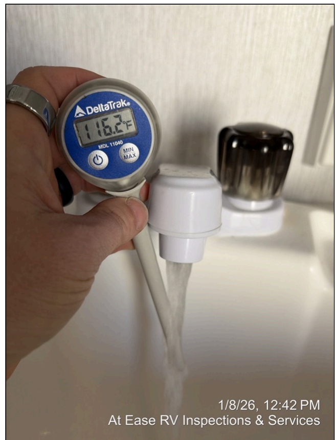
19.23 Item 2 (Picture) Hot water temp
