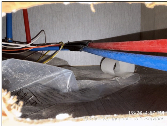
15.9 Item 3 (Picture) Pex line running behind outside fridge2
