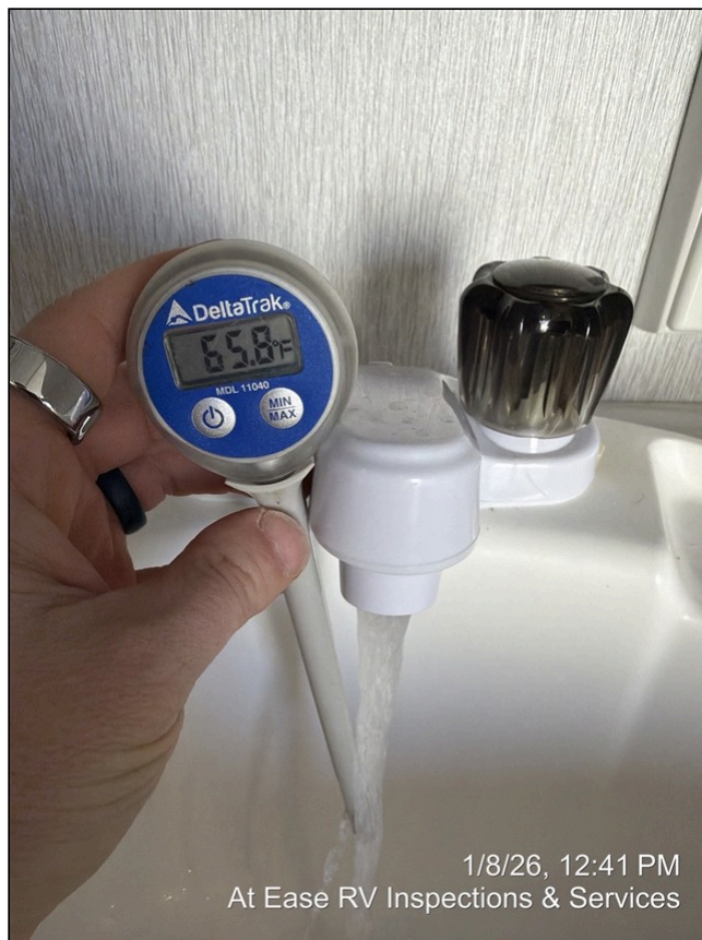
19.23 Item 1 (Picture) Cold water temp
