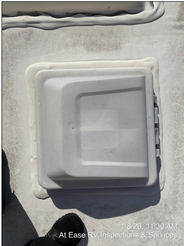
6.6 Item 1 (Picture) Vent
