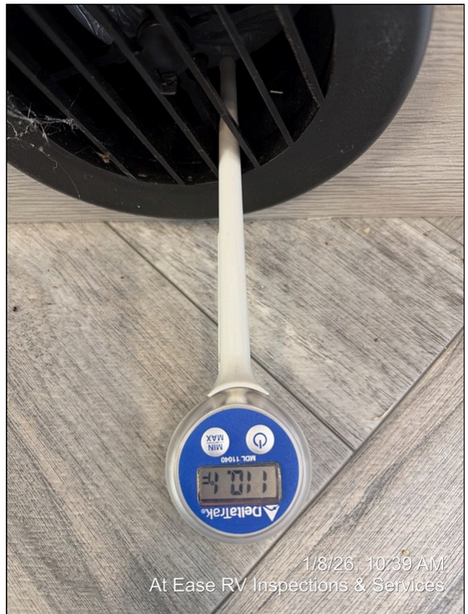
17.10 Item 2 (Picture) Vent by sink
