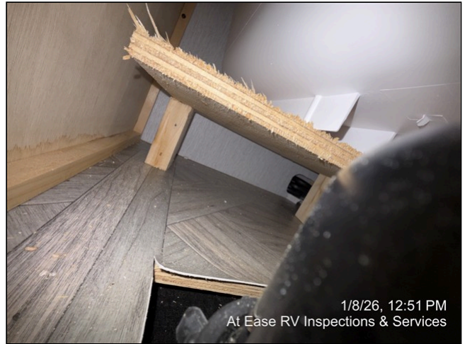
19.17 Item 3 (Picture) Under shower
