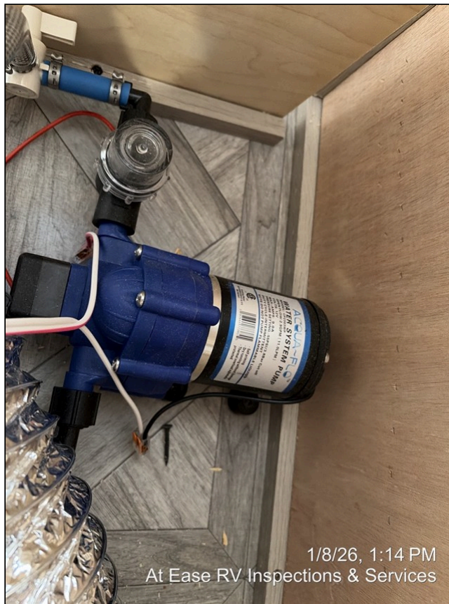
15.9 Item 1 (Picture) Water pump under kitchen sink
