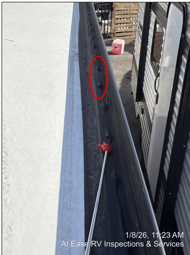
9.2 Item 1 (Picture) Gap in tape
