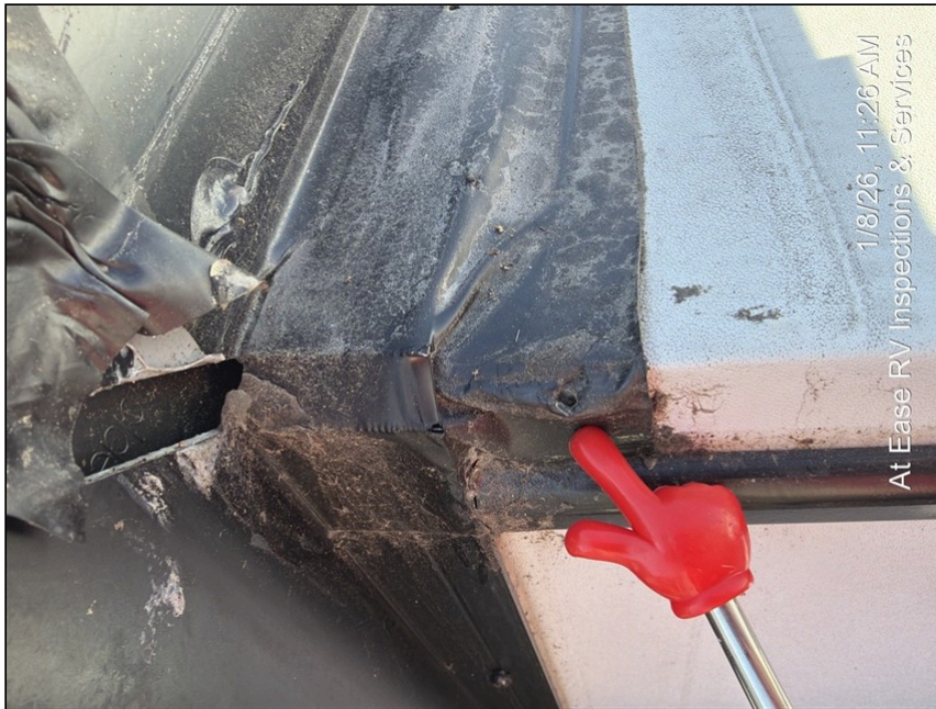
9.2 Item 2 (Picture) Gap in tape
