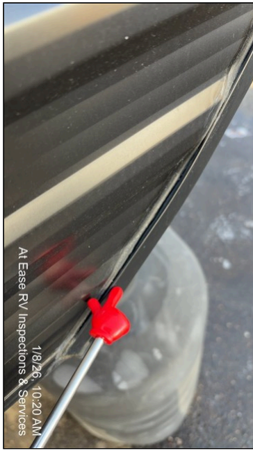
7.2.B Item 1 (Picture) Cracked sealant
