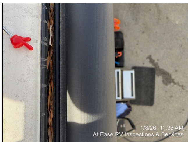
6.0 Item 1 (Picture) Debris in gutter
